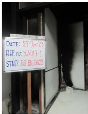
After Fire Test
