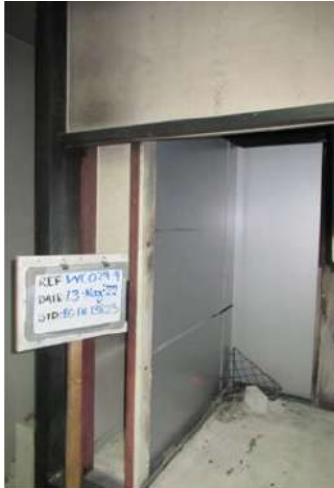
Before Fire Test
