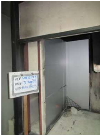
Before Fire Test
